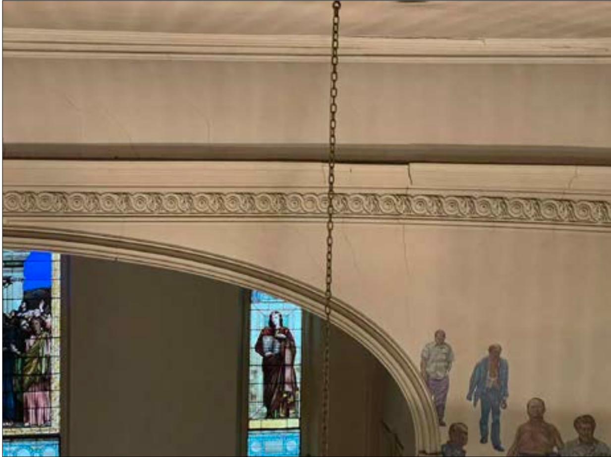
Photo 09. Dislodged molding at belt course above mural and leaded glass. The source of this damage is water penetration at the tower of the Pastor’s Study, which has been restored as a result of the “Opening Doors” campaign. This – and other – large plaster sections are completely disengaged from the wall system.
