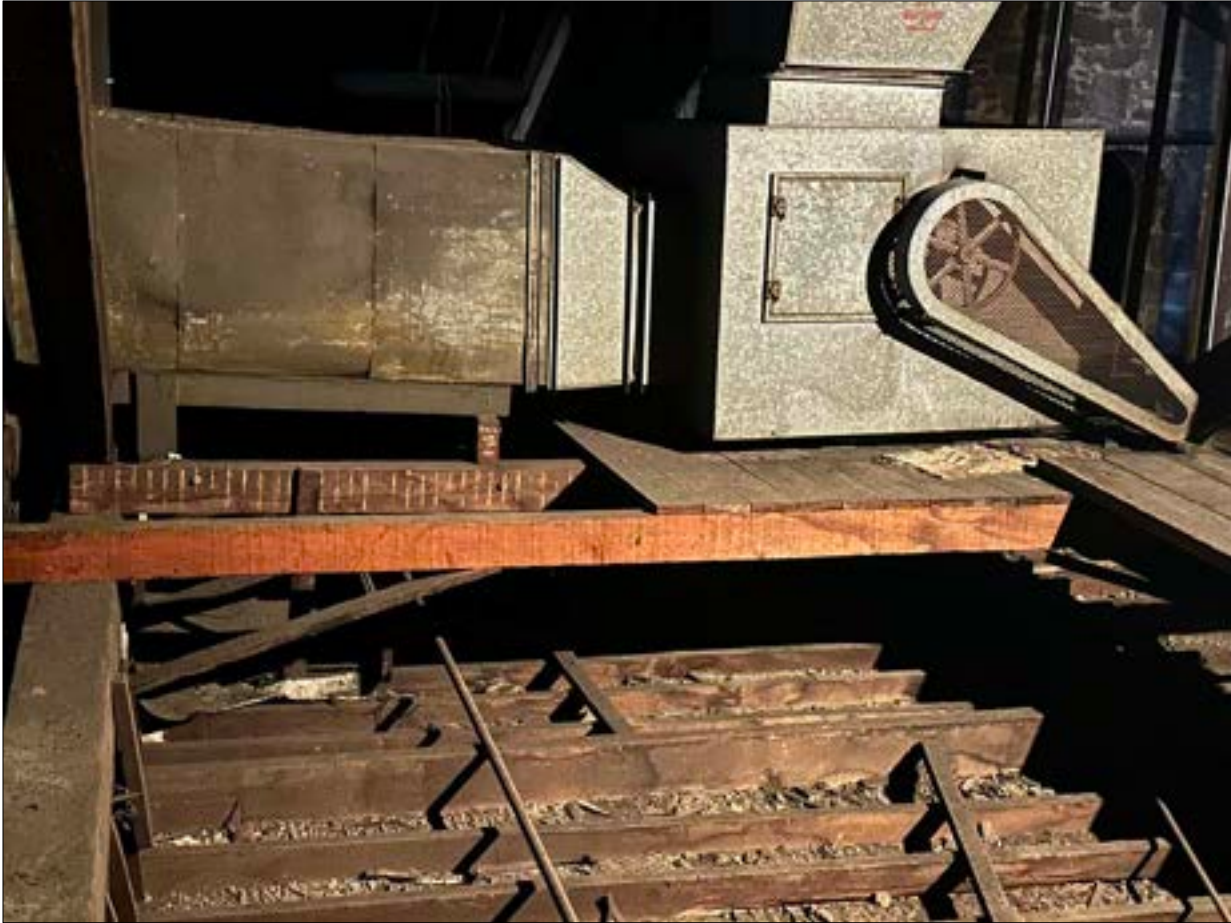
Photo 12. Installation of mechanical equipment introduces a significant level of vibration never intended for this structural system. Aside from drawing large volumes of concentrated air (vs the ambient, more gentle, convective heating/cooling of the 1860s design) inflexible ducted systems present myriad negative issues.
