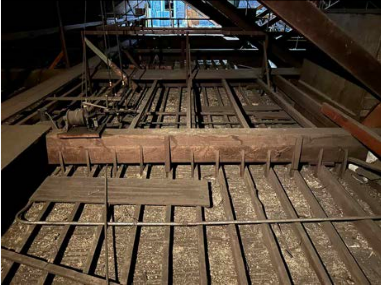
Photo 04. Exceptionally crafted in 1860, the timber & wood framing structural system supporting the ceiling remains in excellent condition; plaster keying through lath, on the other hand, is corrupted in many locations.
