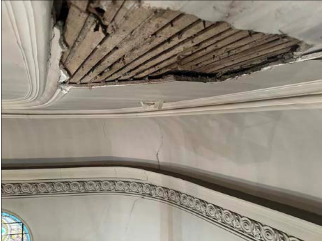
Photo 07. Site of flat plaster failure of August 10-11, 2023, located in the southeast quadrant of the ceiling, above the cove and just east (left) of the organworks.
