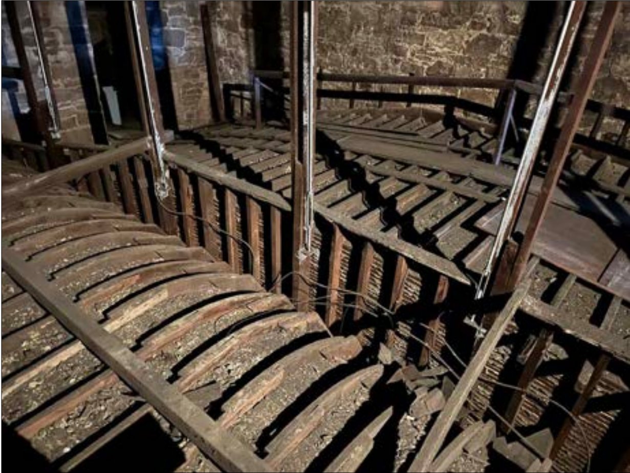
Photo 05. Catwalk over the proscenium arch, where an additional plaster collapse occurred. Concentrated foot traffic in this location renders it more prone to applied forces and, correspondingly, to damage.
