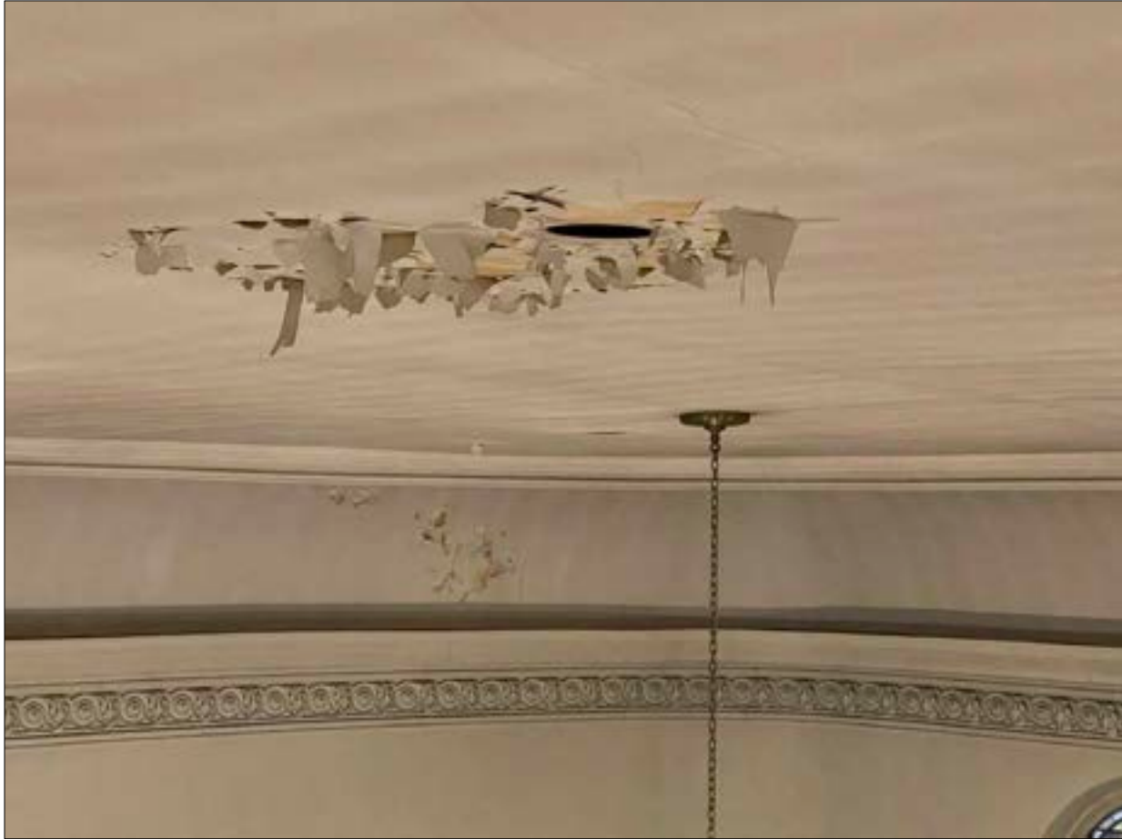
Photo 10. Damage is clearly apparent in the vicinity of all high-hat light fixtures. Reasons include unintended air passage, extreme drying-out because of their heat, and physical damage resulting from their installation.
