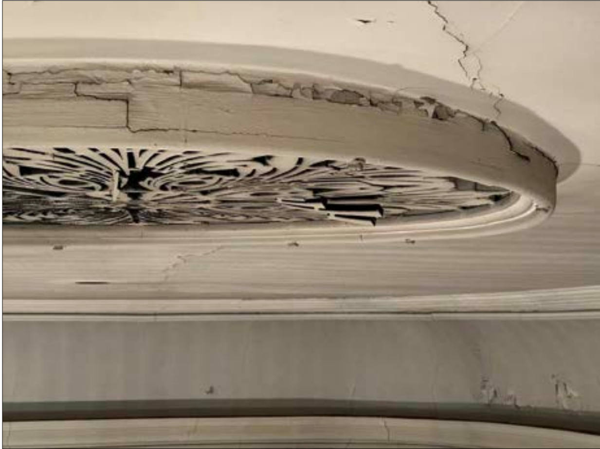
Photo 14. Detail of the molded medallion and vent grille in Photo 13. Note the buildup of infill material applied during the last painting project; this feature was already in a failure mode then.
