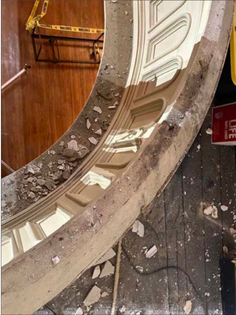
Photo 03. Remnant plaster shards remain scattered in upper reaches of balcony.
