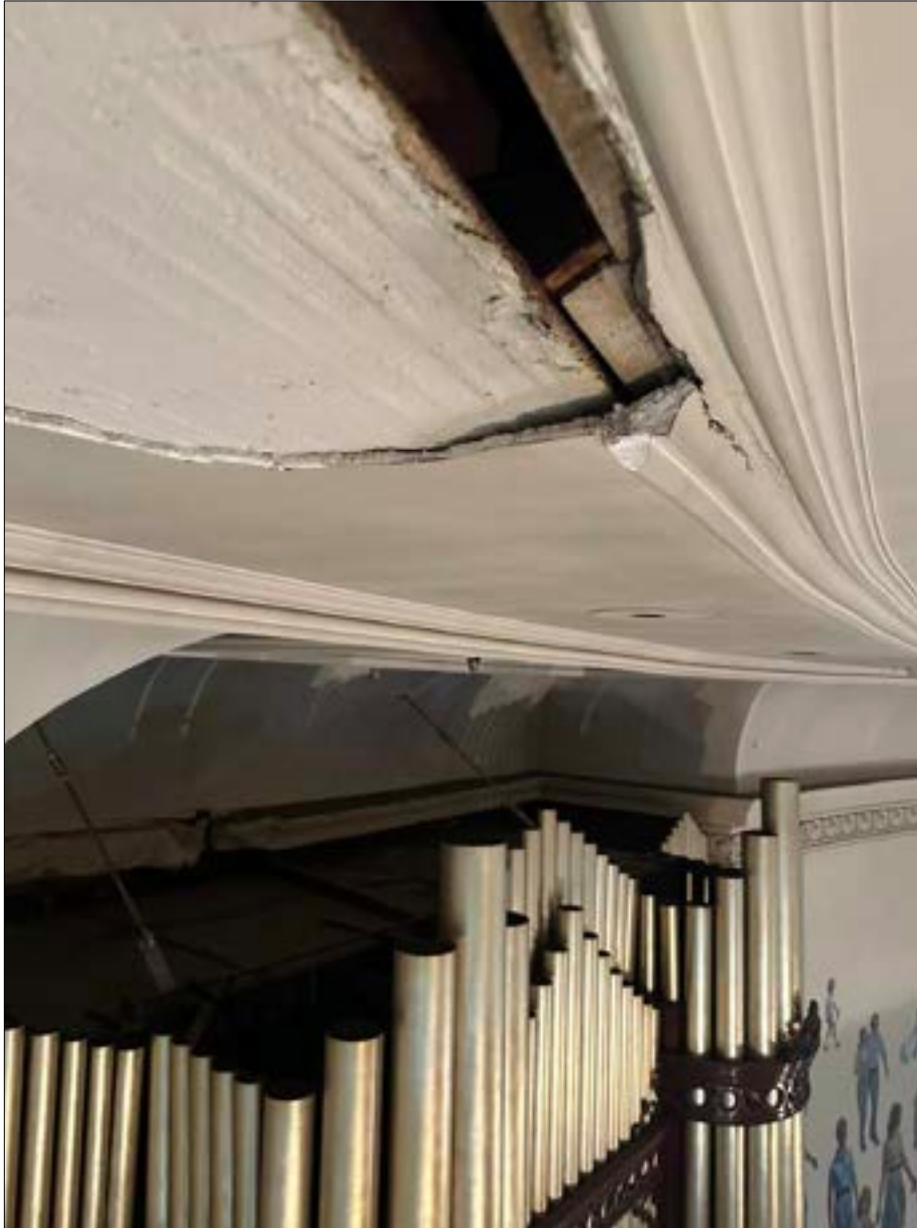
Photo 08. Detail of failure looking west toward organ. The white plane of material represents a flow coat of adhesive applied when the high-hat light fixtures were installed, likely because cracking was evident in the area of the intervention.
