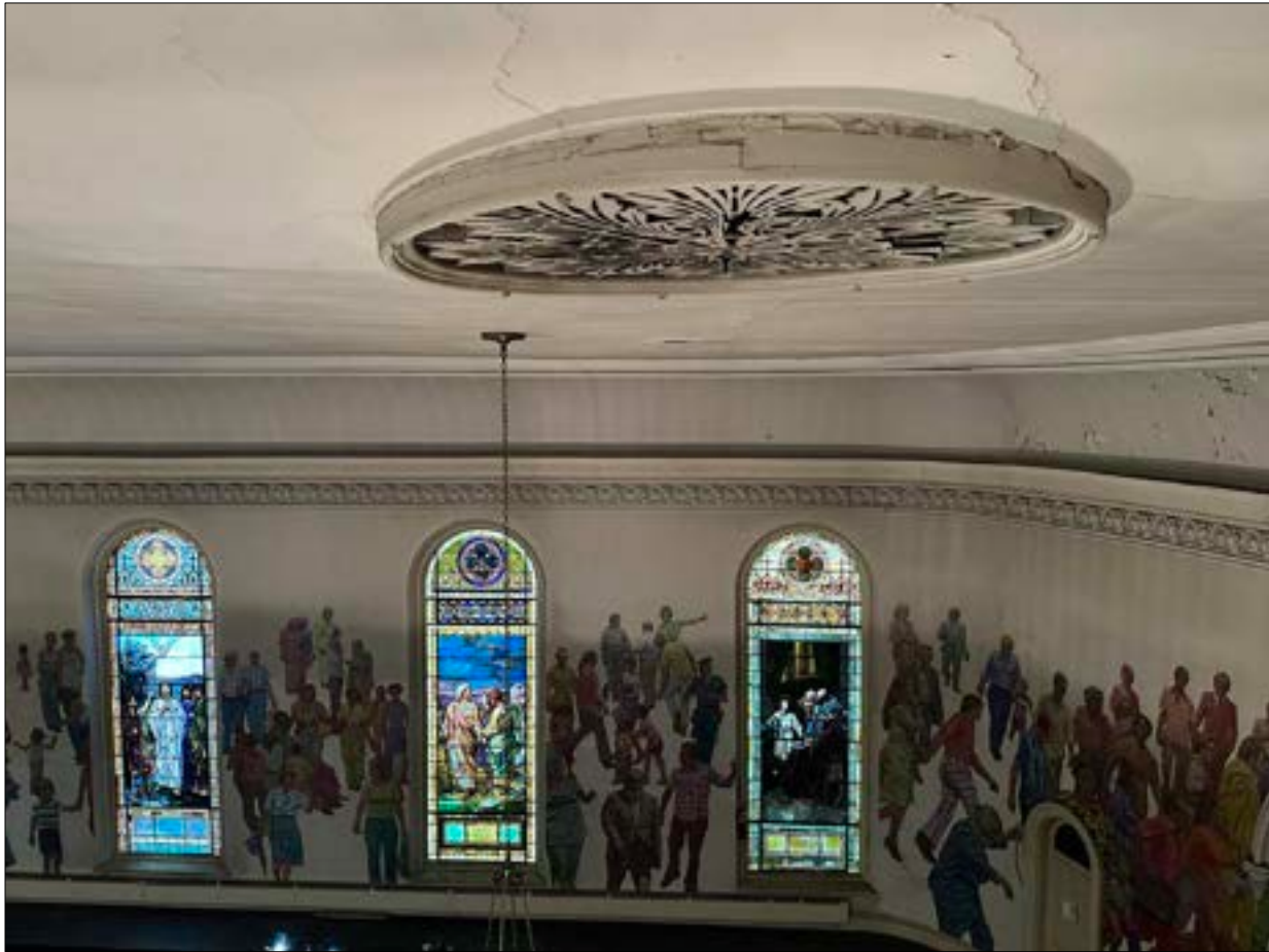
Photo 13. One of three targeted terminals of the ducted system above, deformation and other damage was clearly evident during the last painting campaign, 50-70 years ago. It's gotten worse.
