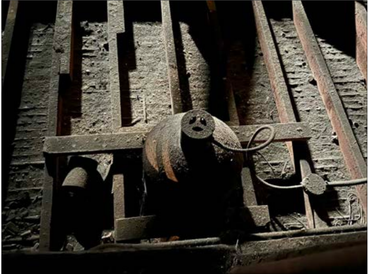
Photo 11. Installation of a high-hat light fixture from above, viewed from within the attic.
